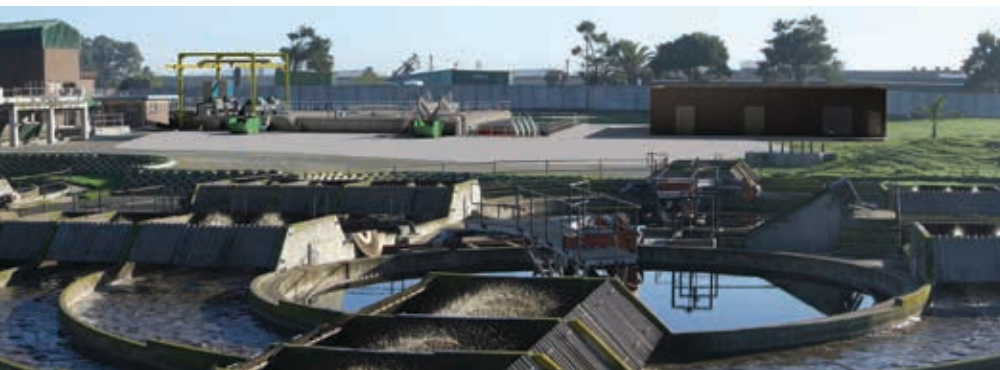
At the Bellville wastewater treatment works, Veolia's membrane bioreactors process 20 Mℓ/day of sewage in a footprint five times smaller than the conventional plant.
